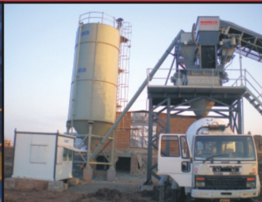
Front view of 90m 3 /hr Plant
