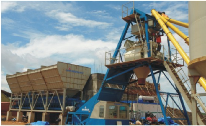
66 m 3 / hr. Plant with Skip & Inline Silo
